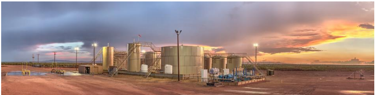
WaterBridge produced water handling facility.
